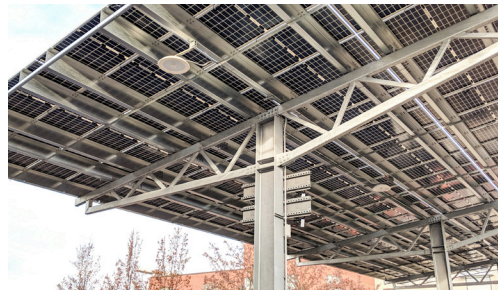
VGBN and the Burlington 2030 District hosted a tour of ECHO's solar parking area adjacent to Lake Champlain in September 2022.
